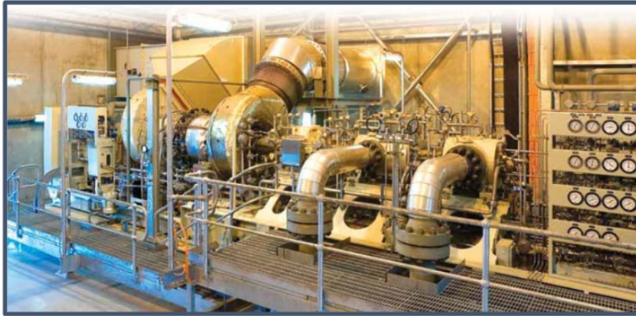
Solar GT driven tandem, skid mounted
